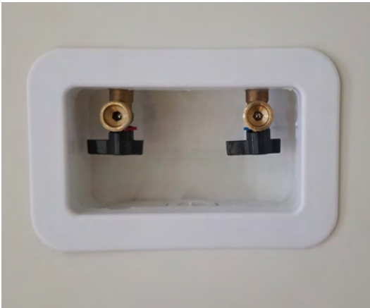
Laundry Machine shut-off valves. Typically located beside or behind laundry machine. Refer to Homeowners Manual for suggested shut off times.
