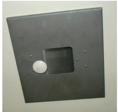
Laundry Room Lint Trap. Typically located above washer/dryer.
